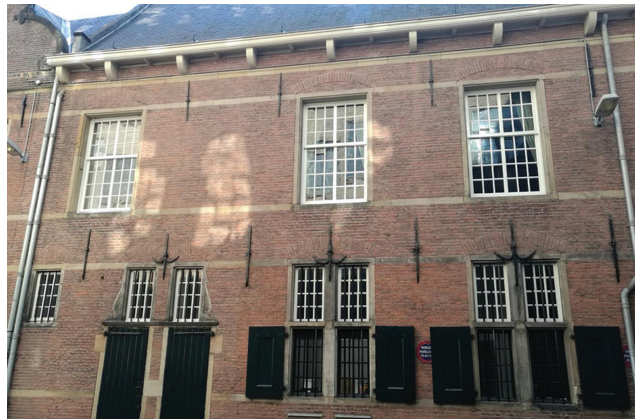
Fig. 20 View of the west wall of the Griffie-building, showing the original muntins on the ground floor. Brick patterns and natural stone ornaments indicate the original window openings, which correspond with the location of the current windows. Photo: A.J.M. van de Meerendonk.
